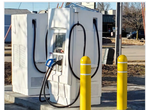
Photo: Level Two and DC Fast Charging Station, Beaver Dam, WI
